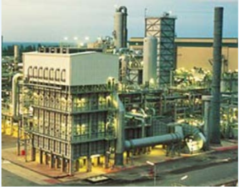
SMR (Steam Methane Reformer)
