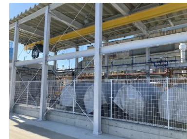
Storage tank for ammonia fuel
